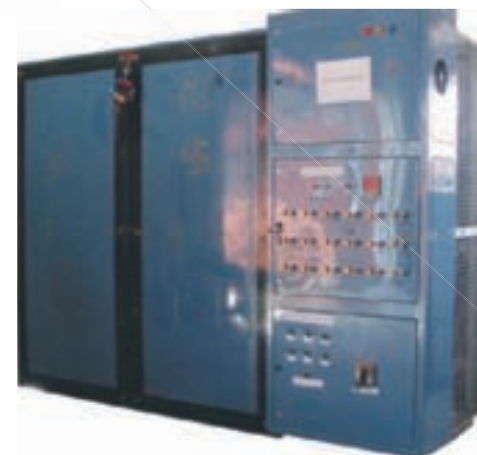
600 KW Generator Load Test Bank
